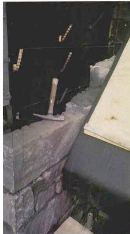
The horizontal string moves up and down. The author set two vertical stringlines at each corner. Between the inside lines he stretched a horizontal line that could be moved up and down on the vertical lines and that established the stone wall's plane. Galvanized metal ties then are nailed into studs.
