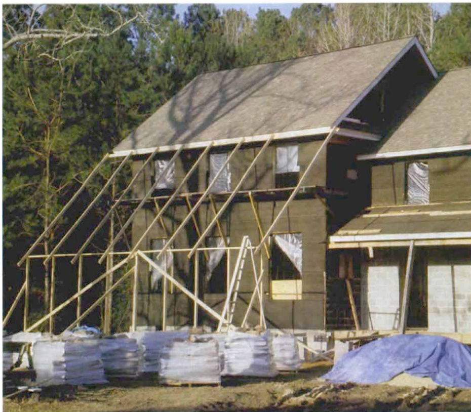
Make a tent to stay dry. A simple 2x4 frame covered with a tarp allows work to move ahead, even during rainy weather. Line run through pulleys at the eaves of the house make raising and lowering the tarp simple.
